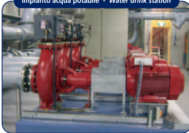
Impianto acqua potabile - Water drink station
